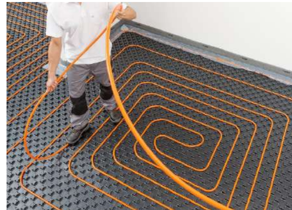
Hot water under-floor heating
